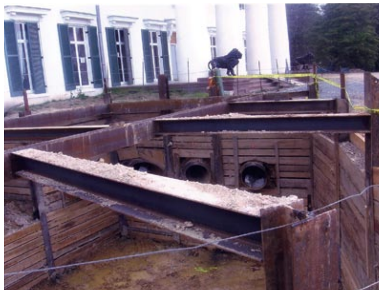
One of the Mansion lions overlooks a section of the intricate shoring and bracing system, including cutouts for utilities, required to support the new geo-thermal HVAC system.
